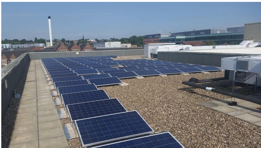
Roof-mounted PV panels at the Maternity Centre at Royal Stoke Hospital
