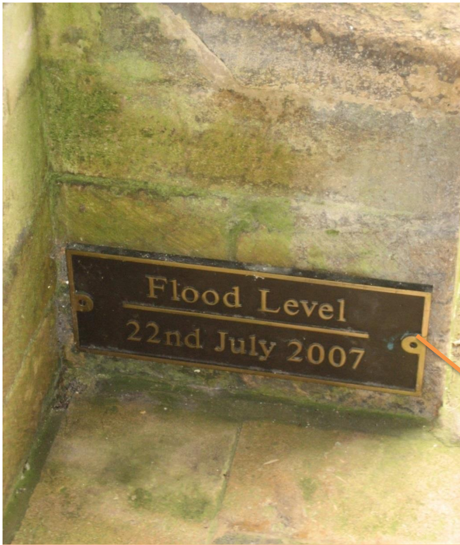
River Severn flood mark, porch to Tewkesbury Abbey, UK
